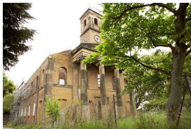
Grade II* Dockyard Church, Sheerness. Burned in 2001. Photo: Kate Peters
