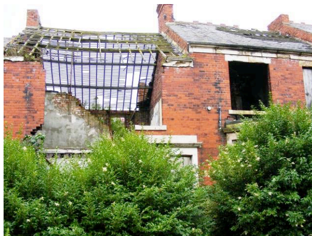
Good housing stock left to decay. Denton, Newcastle
